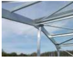
All our buildings are fully braced to BS5950 using rigid bolted components.
